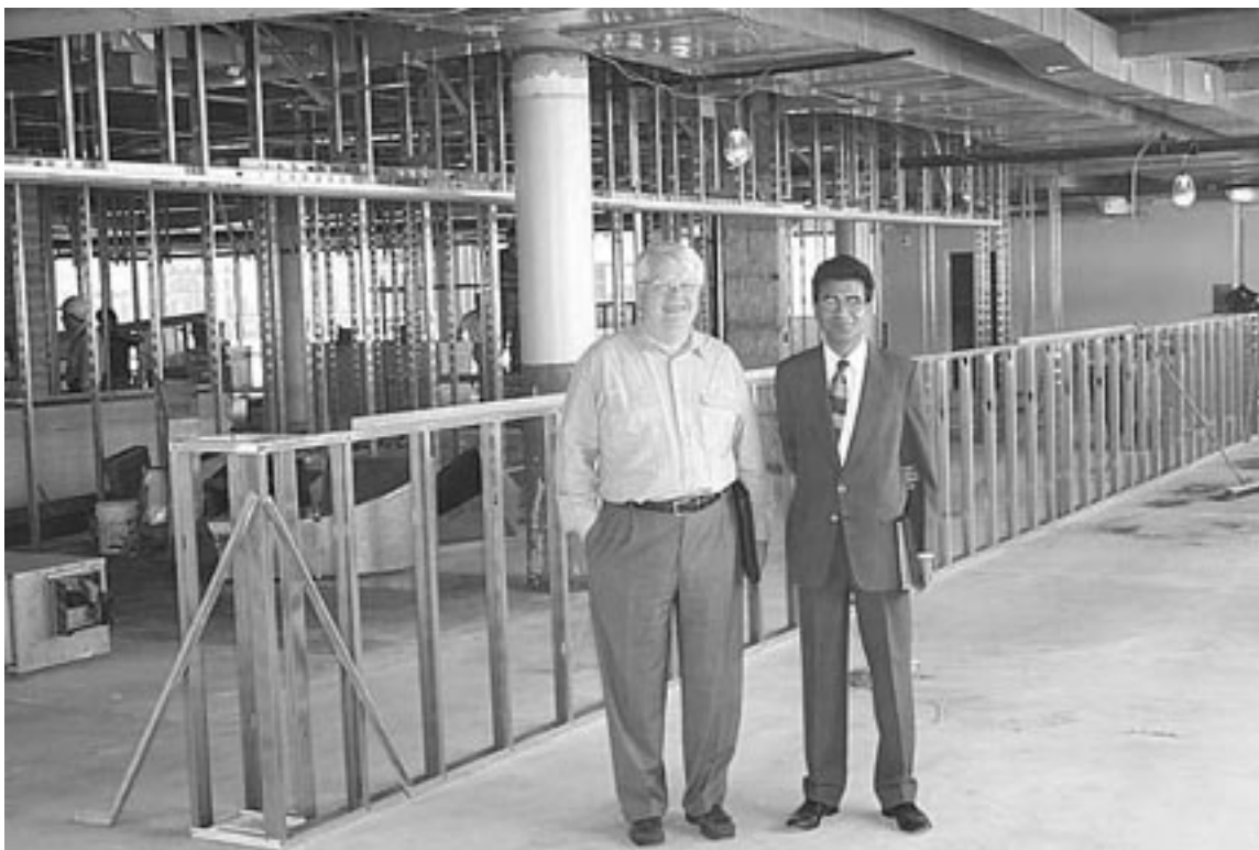
Executive Director Dennis Norlin and Director of Financial Services Pradeep Gamadia inspect progress at ATLA's new headquarters at 250 South Wacker Drive, Chicago.
