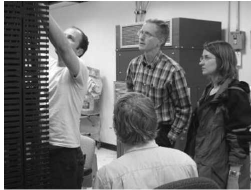
Karl Frantz (center) and Tami Luedtke (right) oversee work in the new server room at 300 South Wacker Drive.
